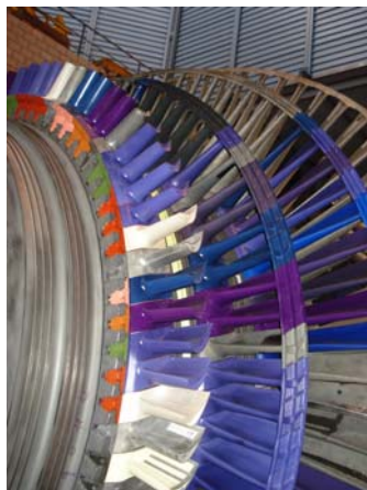
Figure 5.6: GT26 test power plant - thermal paint test of the LP Turbine
