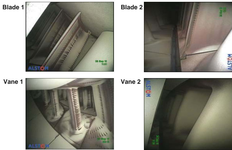
Figure 5.7: LP turbine frontrunner borescope inspection
