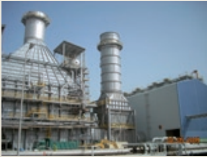
DUBAL GTX EXTENSION UEA 1 x GT13E2 cogeneration – 150 MW
