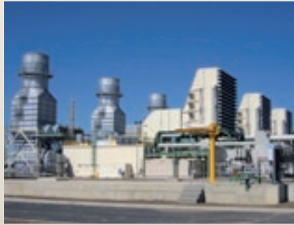
BRAEMER Australia 3 x GT13E2 – 450 MW
