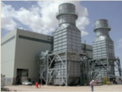
F'KIRINA Algeria 2 x GT13E2 – 292 MW
